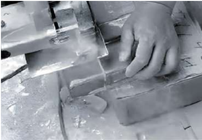
2.4 The modulus of the top layer of bricks is wrong, you can use a diamond saw blade to cut and fill.
